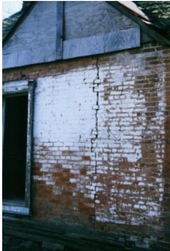
Fig. 10. This crack shows where the east room was added on to the original one-room brick house. The wall was not stuccoed here because it was protected by the kitchen ell.
